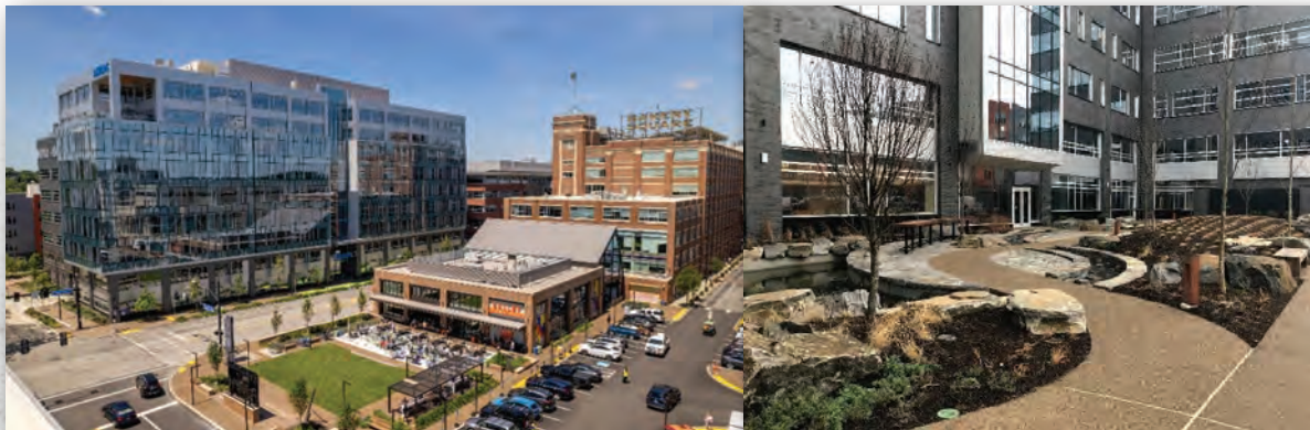
Photos from the 7th Annual Excellence in Concrete Project Award Winner PJ Dick for the Bakery Square Sitework project.
