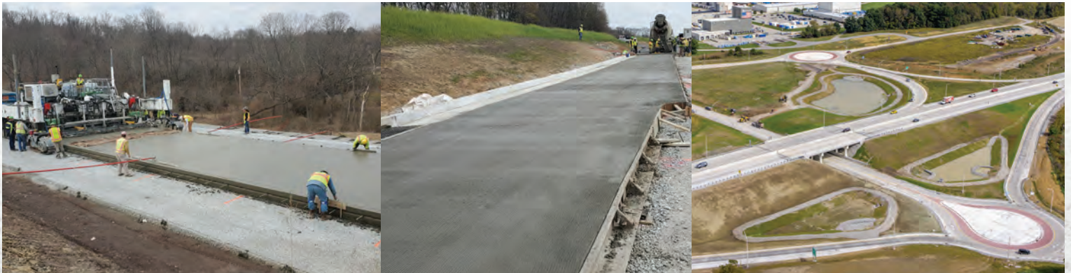
Photos from the 8th Annual Excellence in Concrete Project Award Winner Golden Triangle Construction for the SR70 Yukon & Madison Interchanges project.
