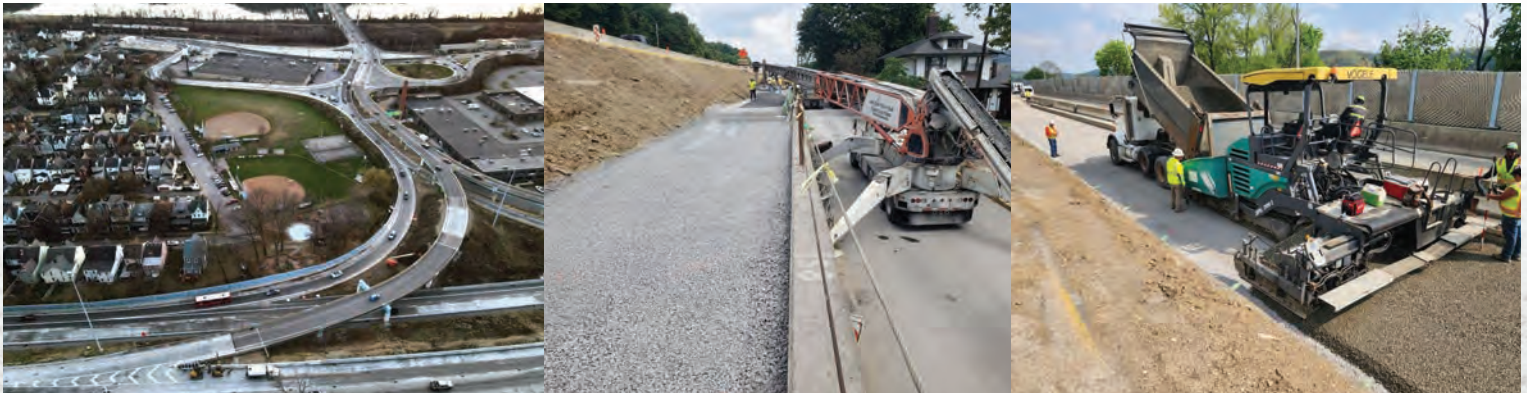
Photos from the 9th Annual Excellence in Concrete Project Award Winner Golden Triangle Construction for the SR28 Highland Park Bridge Interchange project.
