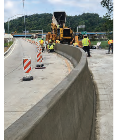
Photo from the 9th Annual Excellence in Concrete Project Award Winner Golden Triangle Construction for the SR28 Highland Park Bridge Interchange project.
